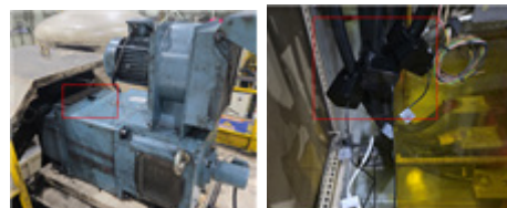
Fig. 1 Vibration&Current Sensors on a Motor
